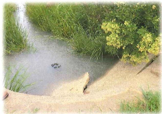
Collapsed headwall at River Road culvert during high tide, approximately 2,000 feet west of Chief Road (OO_04).
