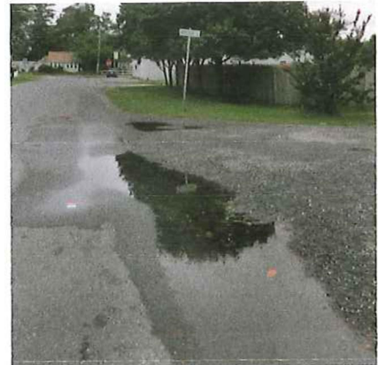
The Intersection of Myrtle Avenue and Delaware Street with standing water
