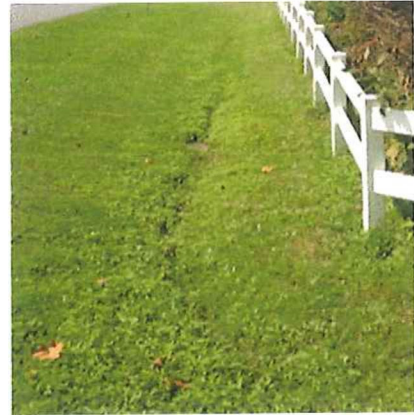
Existing Grass Ditch at the Corner of Oak Orchard Road and Caravel
