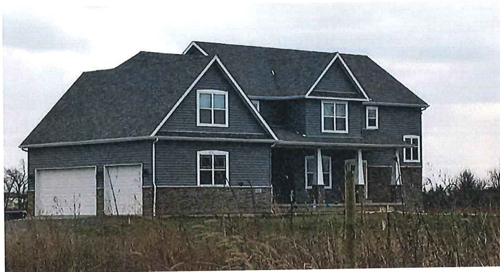
4,255 square foot estate home under construction, adjacent to Portage Solar Farm located in Indiana
