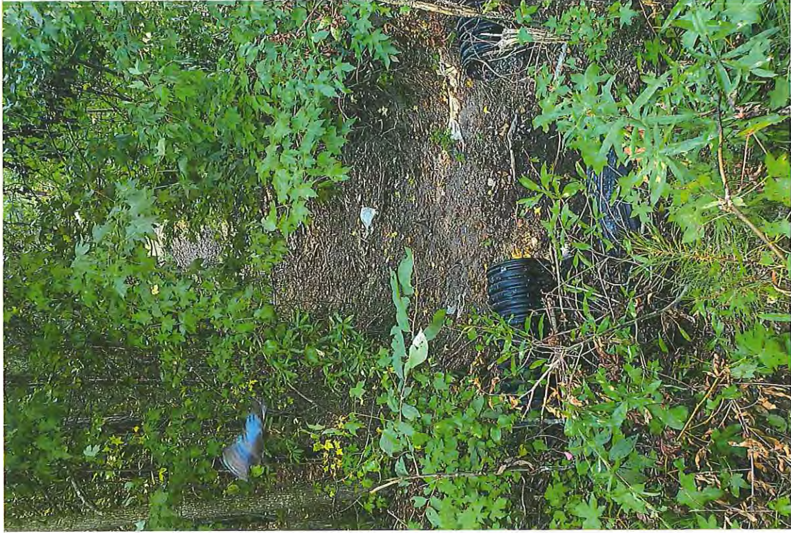
Photo 5 Drainage Channel & Existing Culverts on east edge of farm road to be widened
