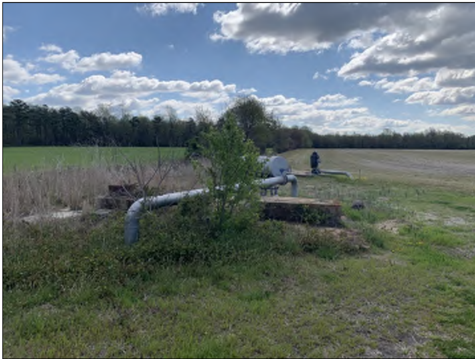
Photograph 6: View of Well Pumping System
