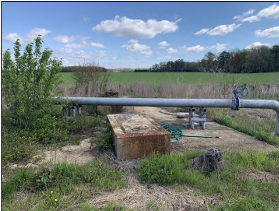
Photograph 8: View of concrete pad that may have once held an AST or Pump
