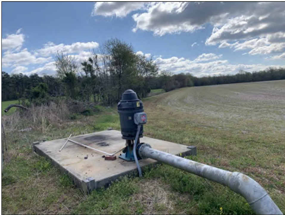
Photograph 10: View of US Motors Electric Well Pump
