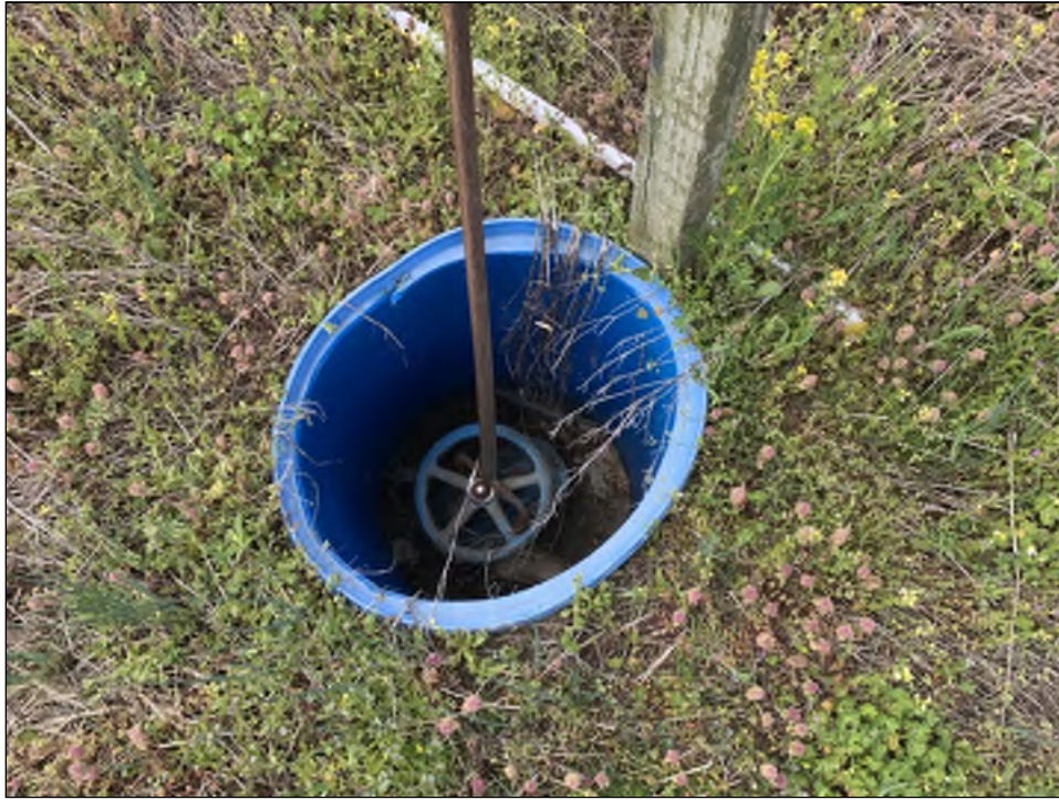
Photograph 11: View of Irrigation Switch
