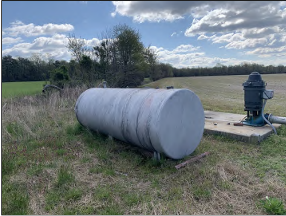
Photograph 9: View of AST adjacent to Well Pump
