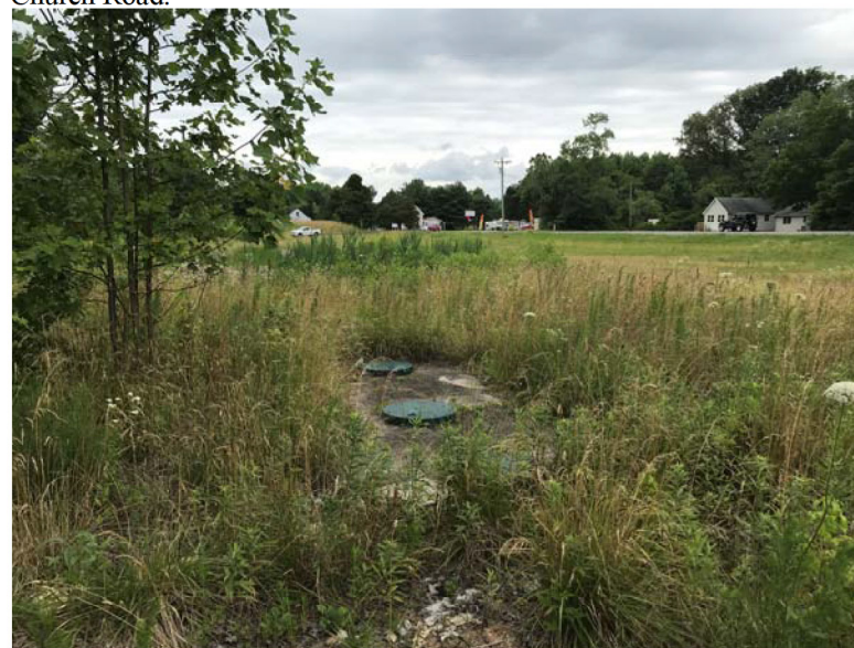
PHOTOGRAPH 4: Apparent tanks associated with wastewater treatment system on the northern portion of the site.
