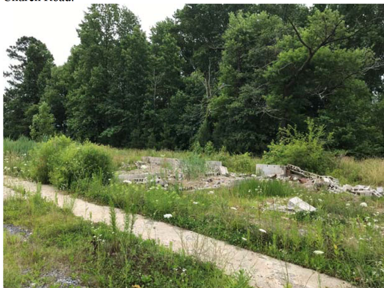
PHOTOGRAPH 3: Debris associated with apparent former apartment structures on the northern portion of the site.
