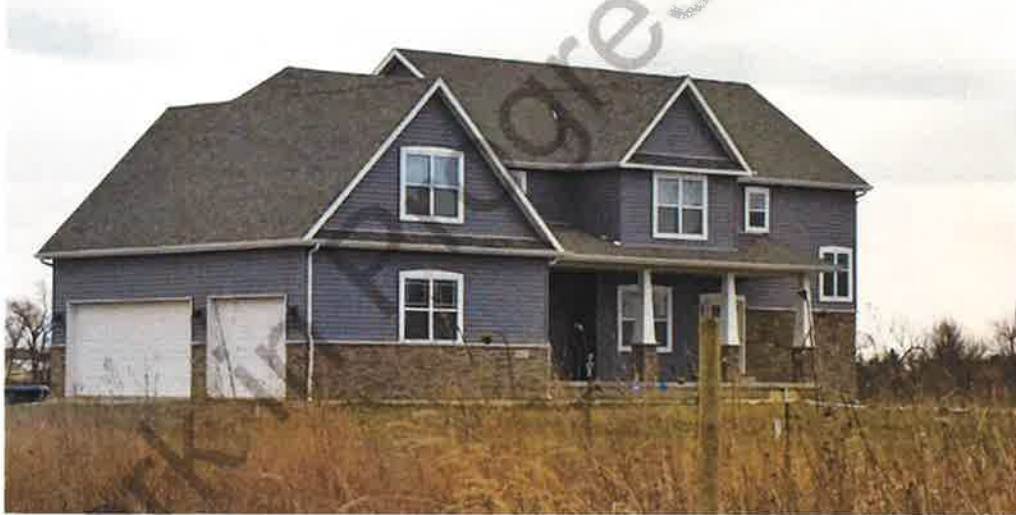
4,255 square foot estate home under construction, adjacent to Portage Solar Farm located in Indiana
