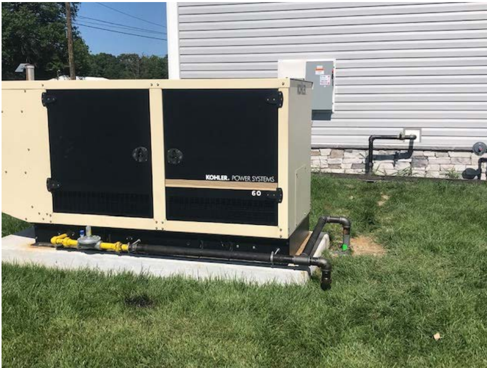
Generator with final natural gas piping configuration
